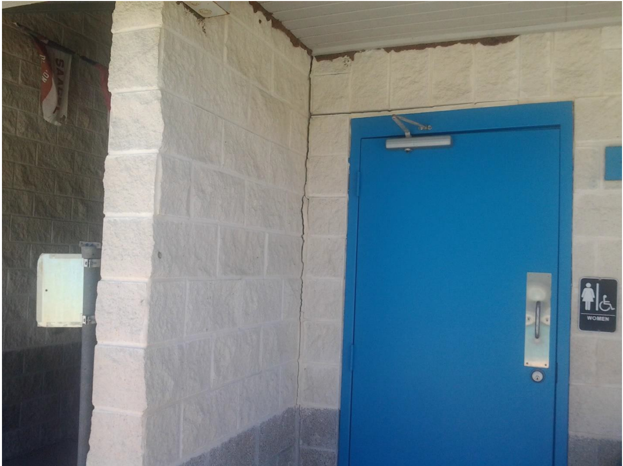
CRACKS IN WALL ENTERING RESTROOM
